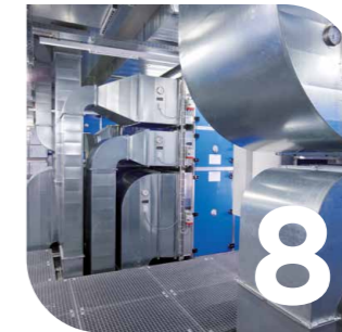
Ventilation and air conditioning
